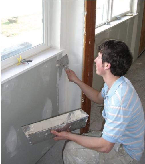
Members of Christian Aid Ministries spent several months assisting Vernonians with home repairs.
