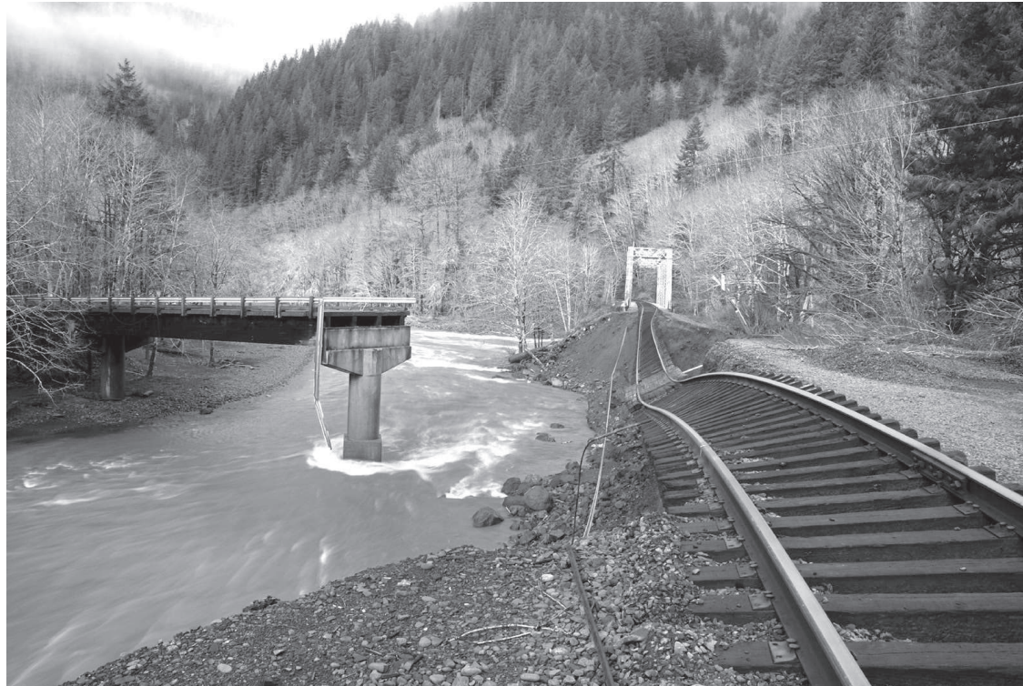
This is an example of some of the damage to the rail line in the Salmonberry River Canyon from the 2007 flood.
