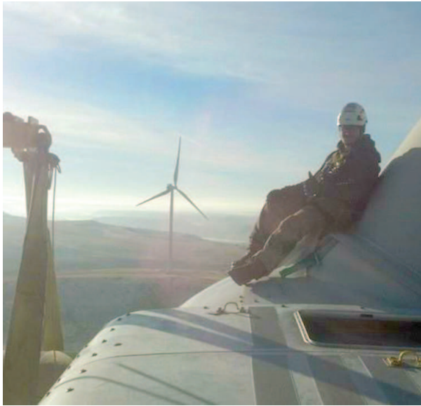
Dillon Dethlefs working on a wind turbine at the Windy Flats Wind Farm in Goldendale, WA.
