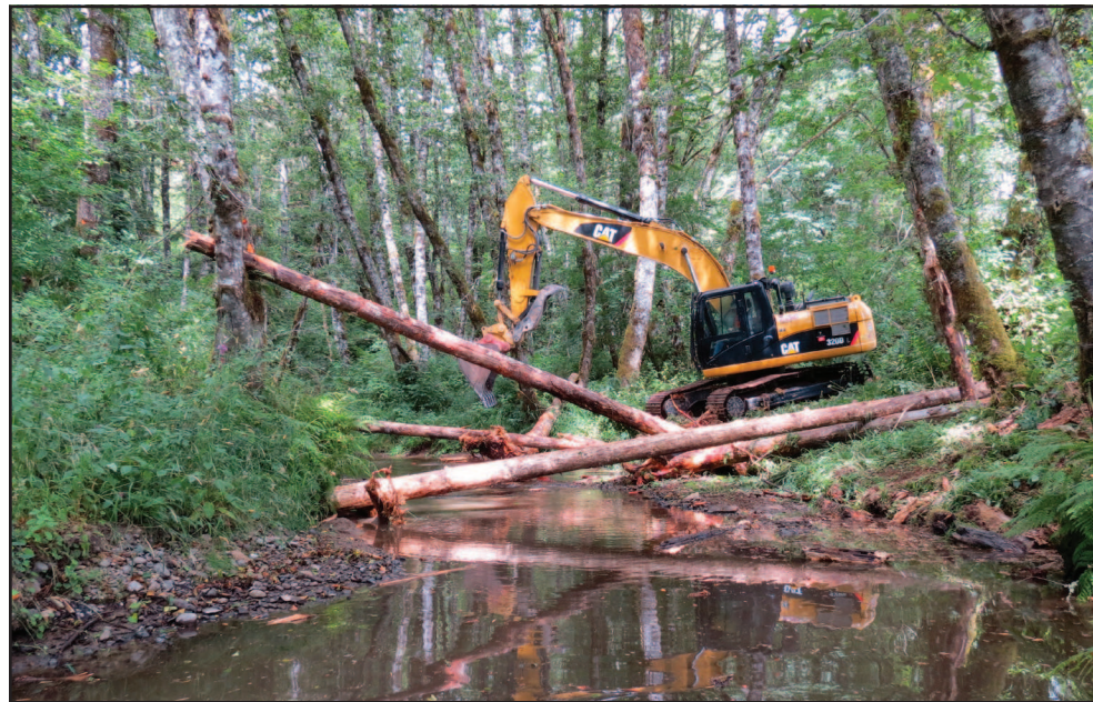
Aquatic Contracting was building salmon habitat on Pebble Creek this past summer.
