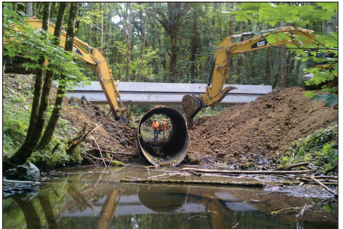
Siegmund Construction removes a culvert to create better fish passage on the Pebble Creek mainline.
