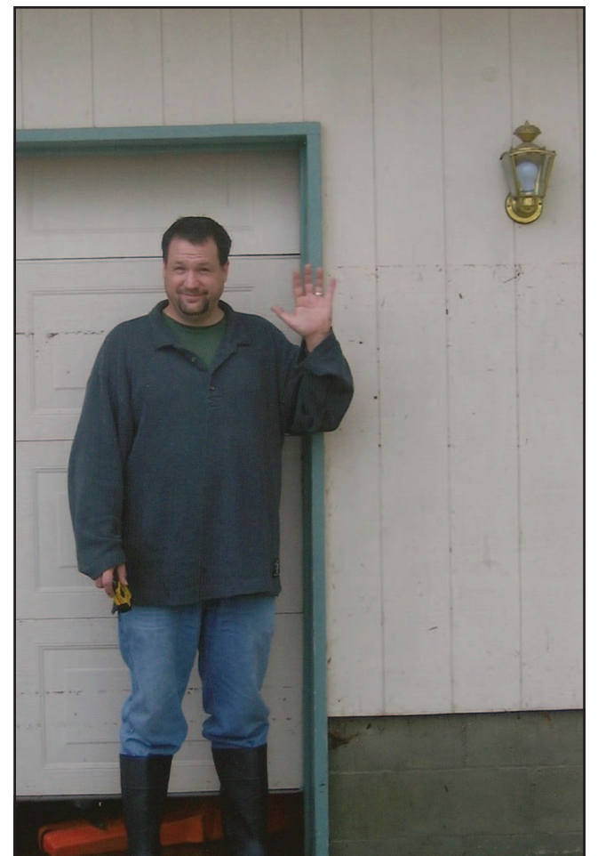
Brandon Eyrrick, who is over six feet tall, stands outside his Juniper Street home; notice the high water line on the wall under the light fixture.
