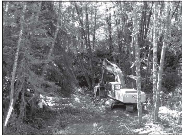
Contractors place large, woody debris into Cold Creek to help create salmon habitat.
