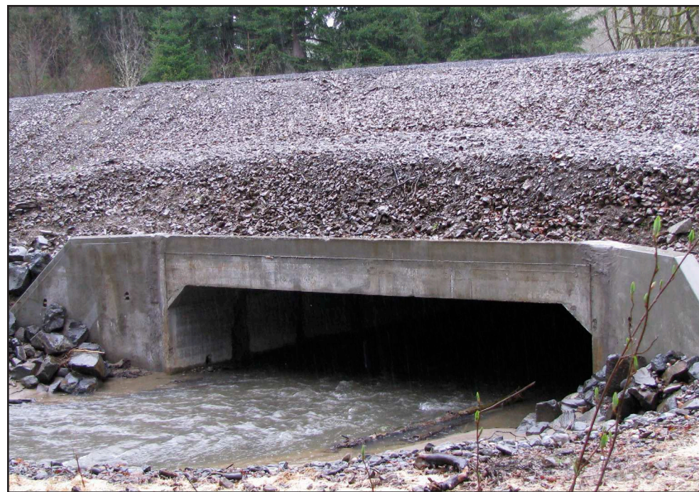
The twenty-four foot wide Elk Creek culvert allows fish to pass under the Scappoose-Vernonia Highway.
