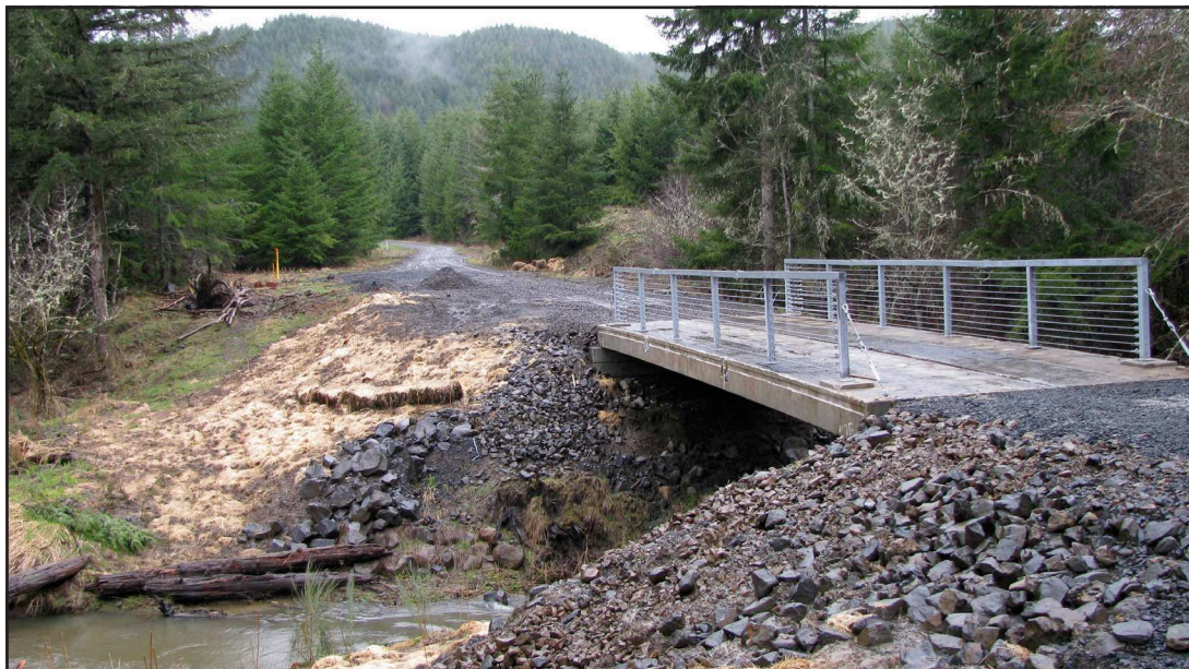
The new bridge on the McKee Mainline, another Project the UNWC helped complete last year.
