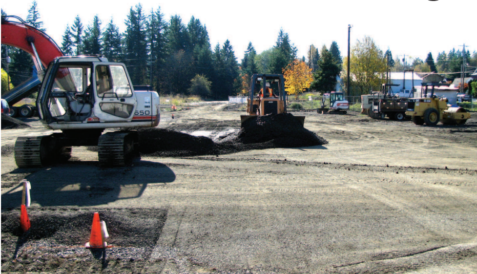
Construction has begun on the new West Oregon Electric Cooperative Headquarters as general contractor Five Star Construction has begun leveling the site.
