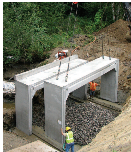
Workers place a new 24 foot wide culvert with a natural stream bed bottom on Elk Creek.
