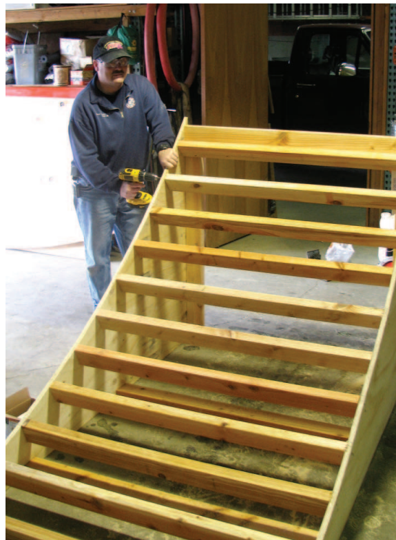
Above: Tom Ramsey builds a skateboard ramp to be installed in the Vernonia Wheels Park. Right: George Tice of the Vernonia Lions Club shows off the site of the temporary Wheels Park.
