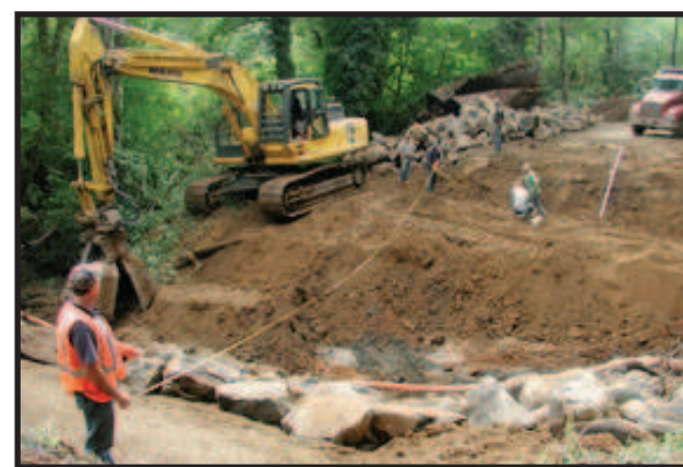
Work crews install a new bridge near Jewell that will allow better fish passage.
