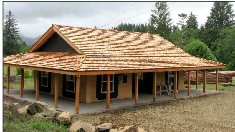
The new Logger Memorial will be housed in this building, currently under construction on the property of the Camp 18 Logging Museum.
