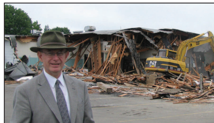
Vernonia Superintendent Ken Cox, as part of the Vernonia high school is demolished
