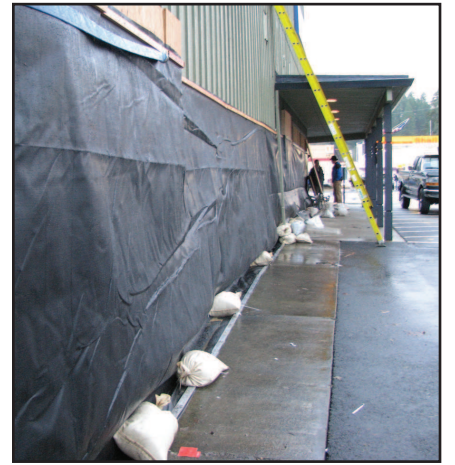
Providence Clinic tried a new idea and "wrapped" their building in an attempt to keep flood waters out.
