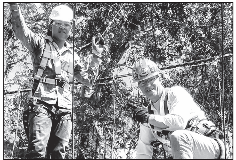
Patrick Montgomery (right), a member of Ironworkers Shopmen’s Local 516 workers with a villager from El Macho, Panama, building a pedestrian bridge across a river that prohibits travel when it rains.
