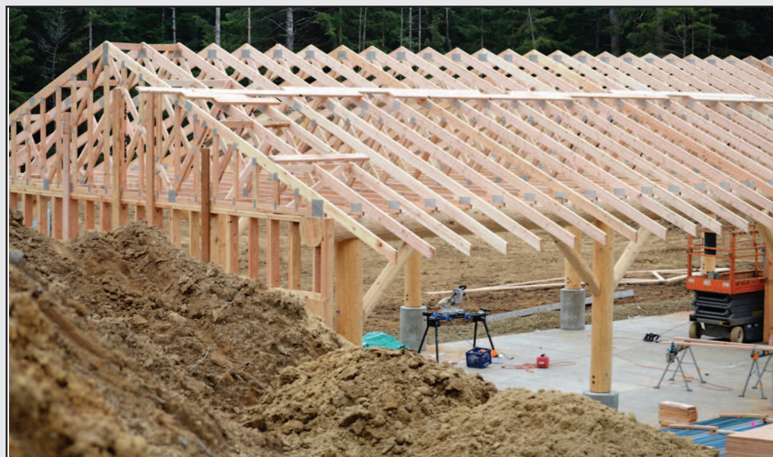
Retired roofer Darrell Hopkins saws plywood sheeting for roof at new shooting sports complex at the Boy Scouts' Camp Meriwether.
