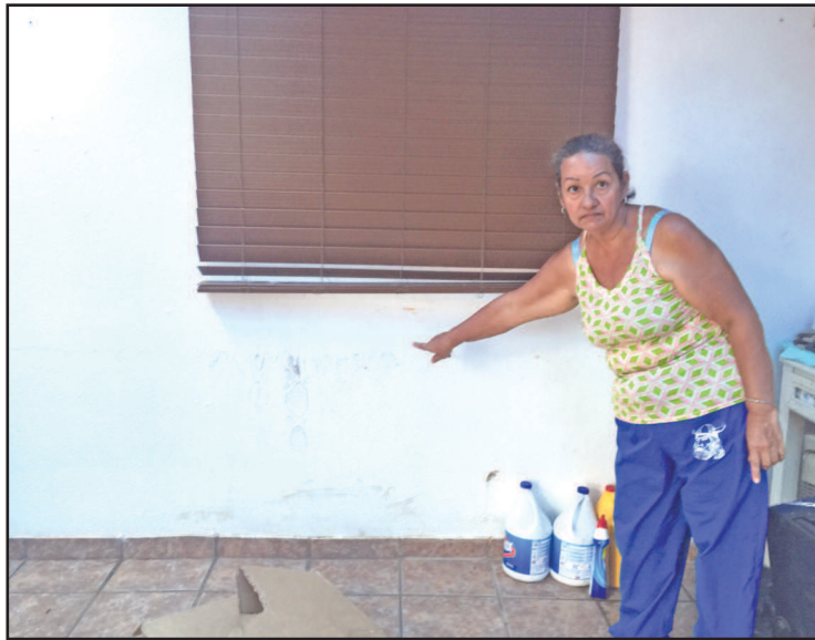
HERE IS WHERE THE WATER CAME ... ON THE SECOND FLOOR. A woman points to a line of black mold, the aftermath of flood waters reached the second story of her home in Barrio Ingenio, half an hour west of San Juan.
