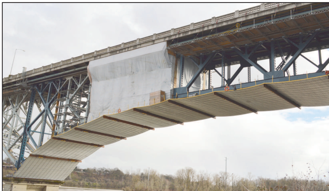
Repainting temporarily halted under Portland's Ross Island Bridge after a 40' fall put two workers in the hospital.
