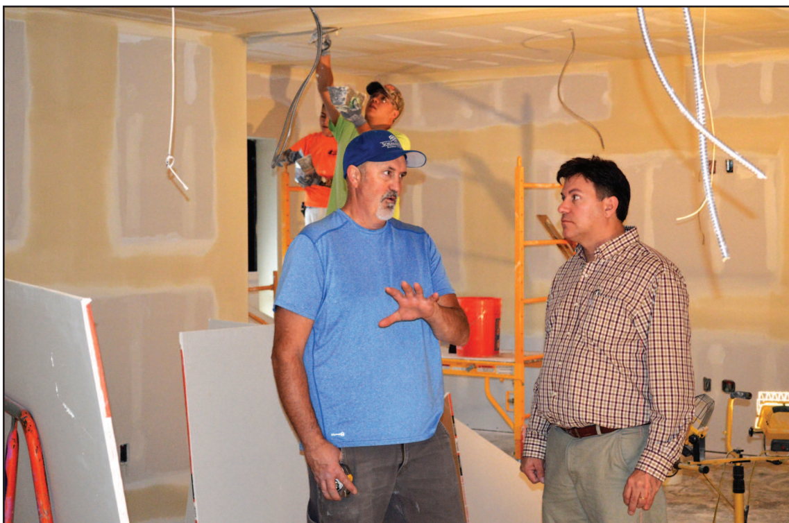
Jim Phelps (right), apprenticeship coordinator for the Painters & Tapers Training Center, talks to Kurt Moore, project manager for Schommer and Sons Construction, as apprentice drywall finishers work in the background.
