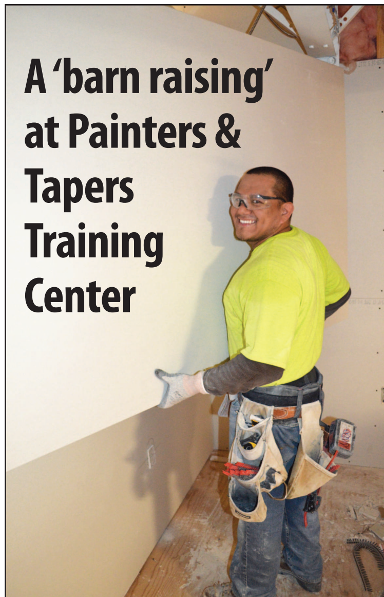
Manny Rodriguez of Performance Contracting (PCI) hangs drywall in a new classroom at the Regional Training Center in Northeast Portland.
