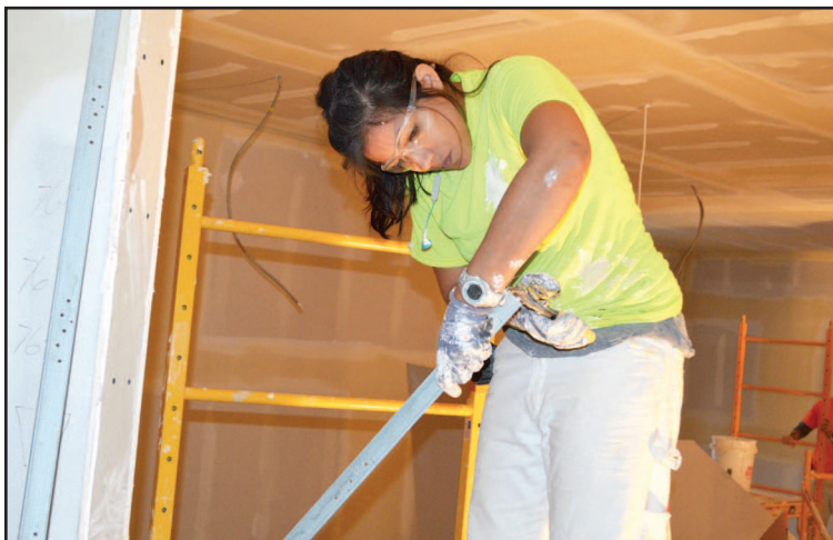
Patricia Gadd, a Level II drywall finisher apprentice and member of Painters and Drywall Finishers Local 10, cuts a metal corner. Gadd works for Harver Company.
