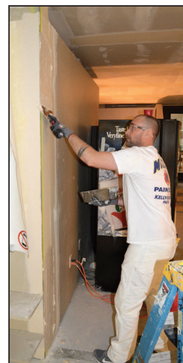
David Adams, a Level III drywall finisher apprentice and member of Local 10, applies a first coat of mud. Adams works for Western Partitions.
