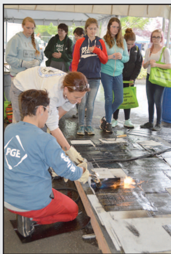
Heidi Kameroff, (leaning forward), a 4th-term apprentice and member of Roofers Local 49, demonstrates "torch down" technique to an interested audience.
