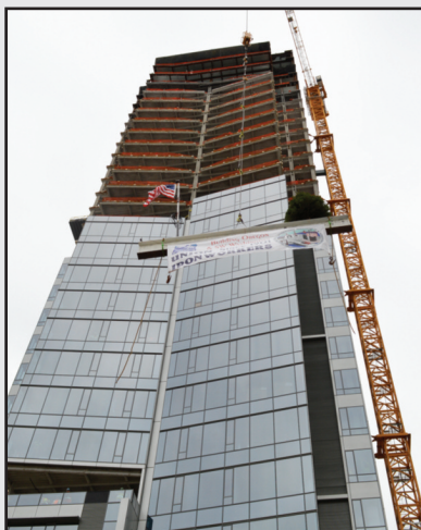
The final beam at Park Avenue West is hoisted into place during a topping out ceremony Feb. 19.
