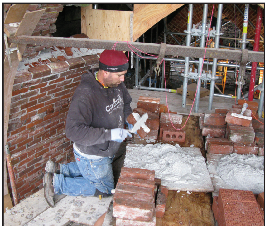
Local 1 member Cameron Orvin restores brick arches inside the furnace to look identical to their original construction.
