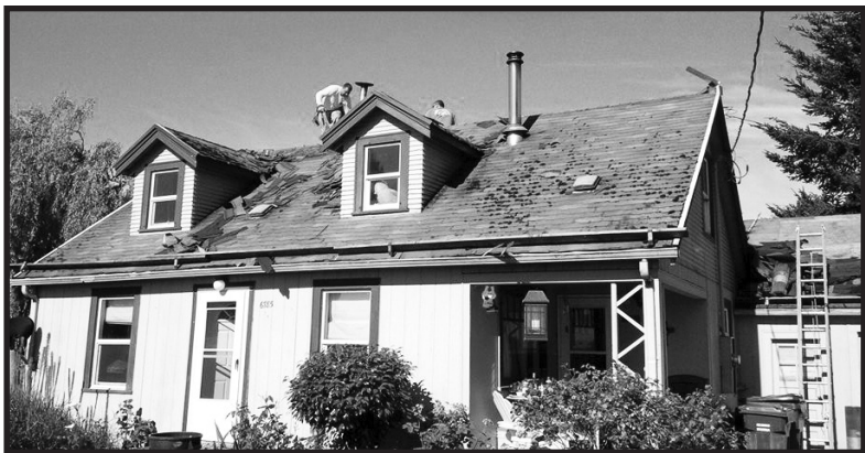
(BELOW) Members of Roofers Local 49 re-roof the home of an injured veteran in Keizer. The soldier did three tours of military duty in the Middle East's war on terror.
