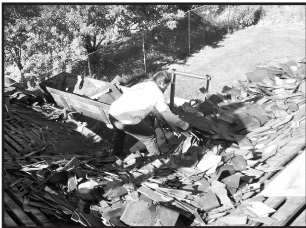
(ABOVE) Roofers Local 49 Recording Secretary Sean Maybee is buried in debris.
