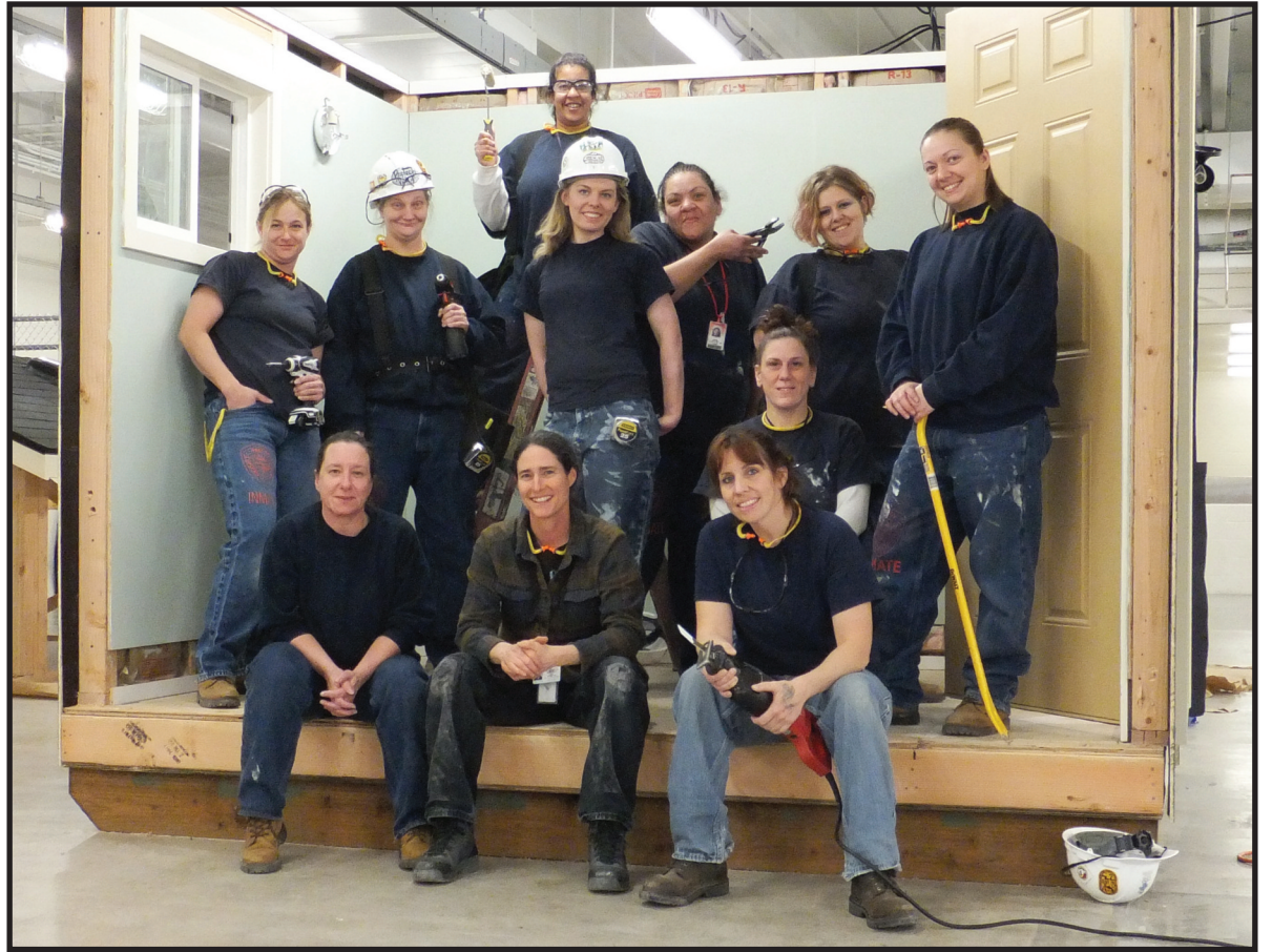
Women inmates at Coffee Creek Correctional Facility fill the partially completed hut they constructed under the direction of vocational instructor Jen Netherwood (front and center). Standing on a ladder at the back is Monica Heusel. Standing, from left, are Charity Henshaw, Gloria Friedrich, Bell Andersen, Molly Lewis, Danelle Klein, and Valayshea Shaffer. Kneeling is Kelly Kissell. Sitting are Tami Johnson, Netherwood, and Shelly McGinnis. (Photo by Dave Conway, general manager, Oregon Corrections Enterprises)
