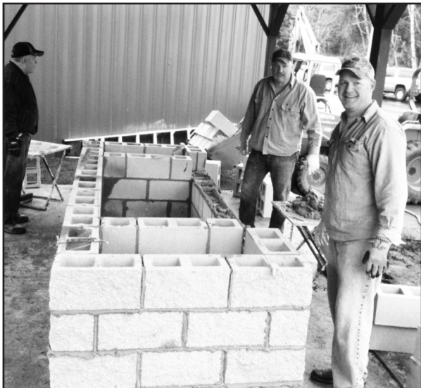
Bricklayers Local 1 Business Agent Mike Titus (left) and Apprenticeship Coordinator Shawn Lenczowski place blocks on new barbecue.
