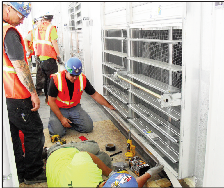
Curtis Cole (left), Tom Boyhan (center), and Brian Rutheford (lying down), members of Plumbers and Fitters Local 290 employed at Temp Control Mechanical, work on the first of three data centers built by Facebook in Prineville. In the background are Rich Schlegal and Aaron Hanlon, electricians for Electrical Construction Co. and members of IBEW Local 280. (Photo courtesy of Facebook)
