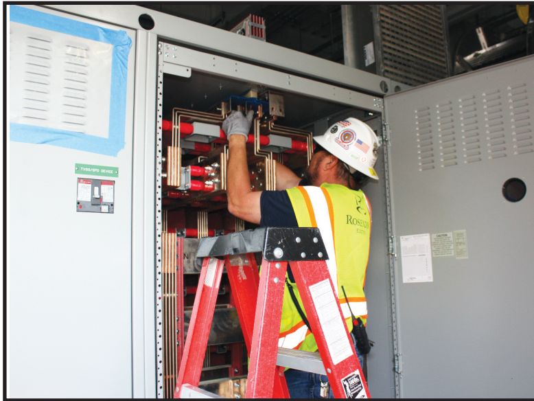
Mike Baker, a member of IBEW Local 280 employed at Rosendin Electric, installs a buss fuse at Building 1 of Facebook's data center complex in Prineville.
