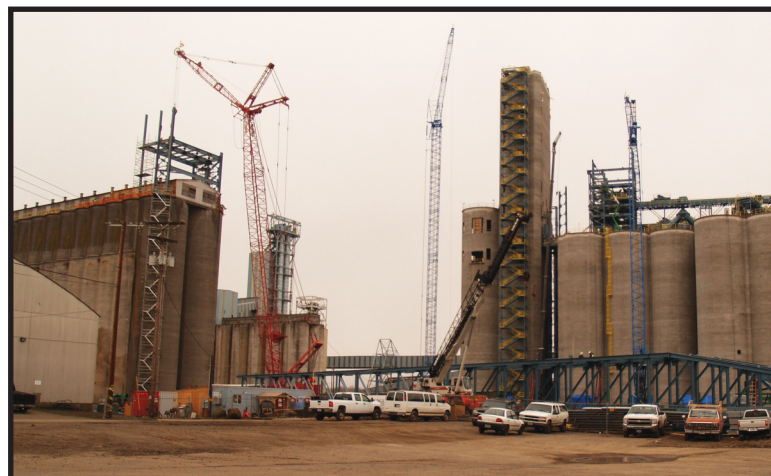
United Grain is constructing an $80 million expansion to its export terminal at the Port of Vancouver.
