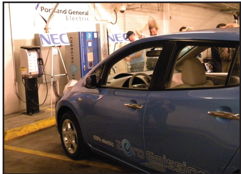
The first public-use electric vehicle charger in the country was installed by union electricians working at Hughes Electrical Contractors. The charging station is located at the World Trade Center parking garage in downtown Portland. Getting amped up for a test drive by Gov. Ted Kulongoski is a Nissan LEAF, an all-electric vehicle coming soon to the Portland market.
