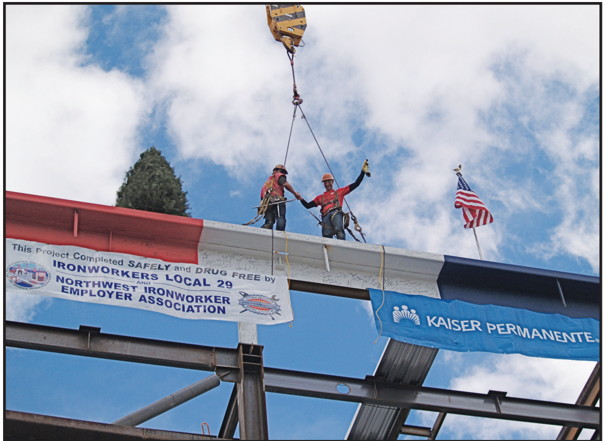
Chris Aldrich (left) and Giles Phillips shake hands after connecting the last iron beam at the Kaiser Westside Medical Center in Hillsboro. The two connectors are members of Iron Workers Local 29 employed at The Erection Company. Kaiser Permanente and the Iron Workers held a "topping out" ceremony April 12. Topping out is a tradition of the union that signifies the completion of a building's structure and to bring good luck. Hoisting the beam into place was Dan Thompson, a member of Operating Engineers Local 701.
