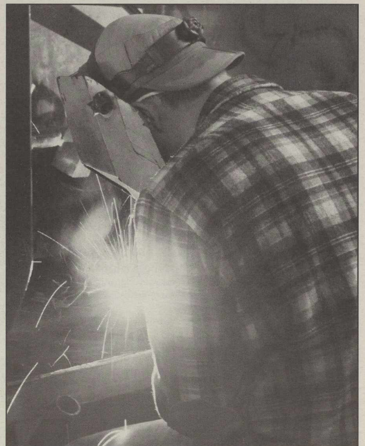
Photo by Laurel Massaro A student in Mylan Rakich's Introduction to Welding class watches sparks fly while welding April 22 at Clackamas Community College. In the past few years, schools like CCC and PCC have begun offering more specialized training classes similar to welding.
