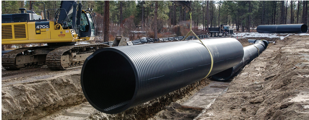
Excavation crews place a section of pipe in the Tumalo irrigation canal. A federal judge has rejected arguments that replacing open canals with pipelines violates an easement across the properties of project opponents.
