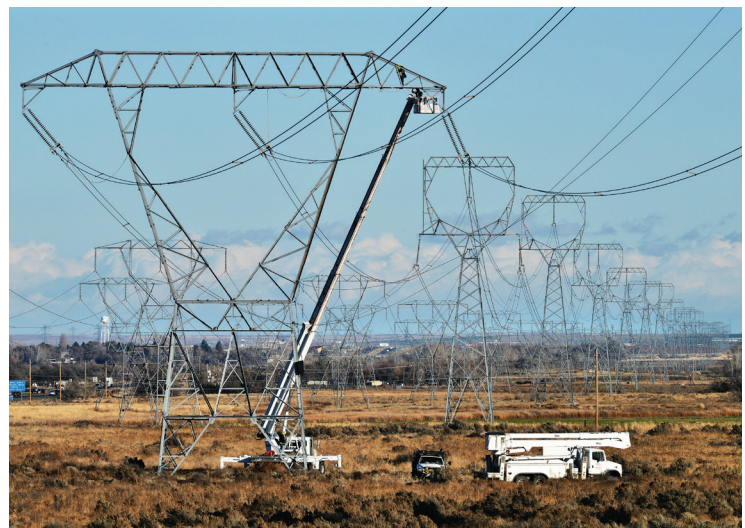
EO Media Group File A crew works on a transmission line tower outside Boardman, Ore. A federal judge has rejected a lawsuit seeking to invalidate the government's right-of-way for the Boardman-to-Hemingway transmission line across public land.
