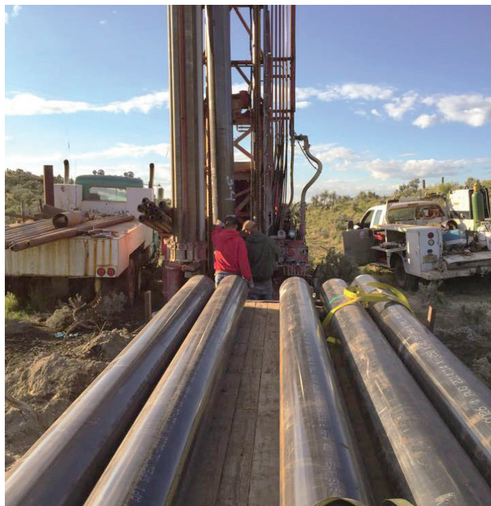
A water well site under construction. About 80% of new wells in Oregon are approved in areas of groundwater concern, according to state water regulators.
