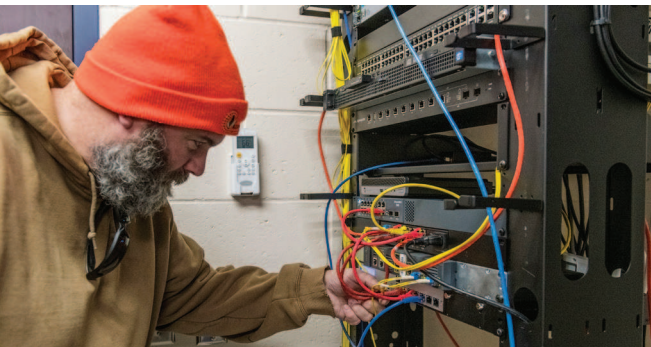
Darrell Hoemann/Midwest Center for Investigative Reporting Tristan Johnson, owner of Wireless Data Net, shows where his system links into the fiber at Blue Ridge High School in Farmer City, Ill. Wireless Data Net is based out of Saybrook, Ill., and serves just under 1,000 customers in 20 smaller rural towns in central Illinois. The company puts its towers on grain elevators and water towers to reach internet customers through its wireless network.
