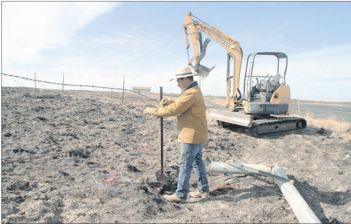
Mario Trejo fixes King Ranch fencing burned in the Grass Valley Fire on Aug. 11 in northern Douglas County, Wash. The fire burned approximately 300 miles of fencing that will cost $4.5 million to $7 million to replace.
