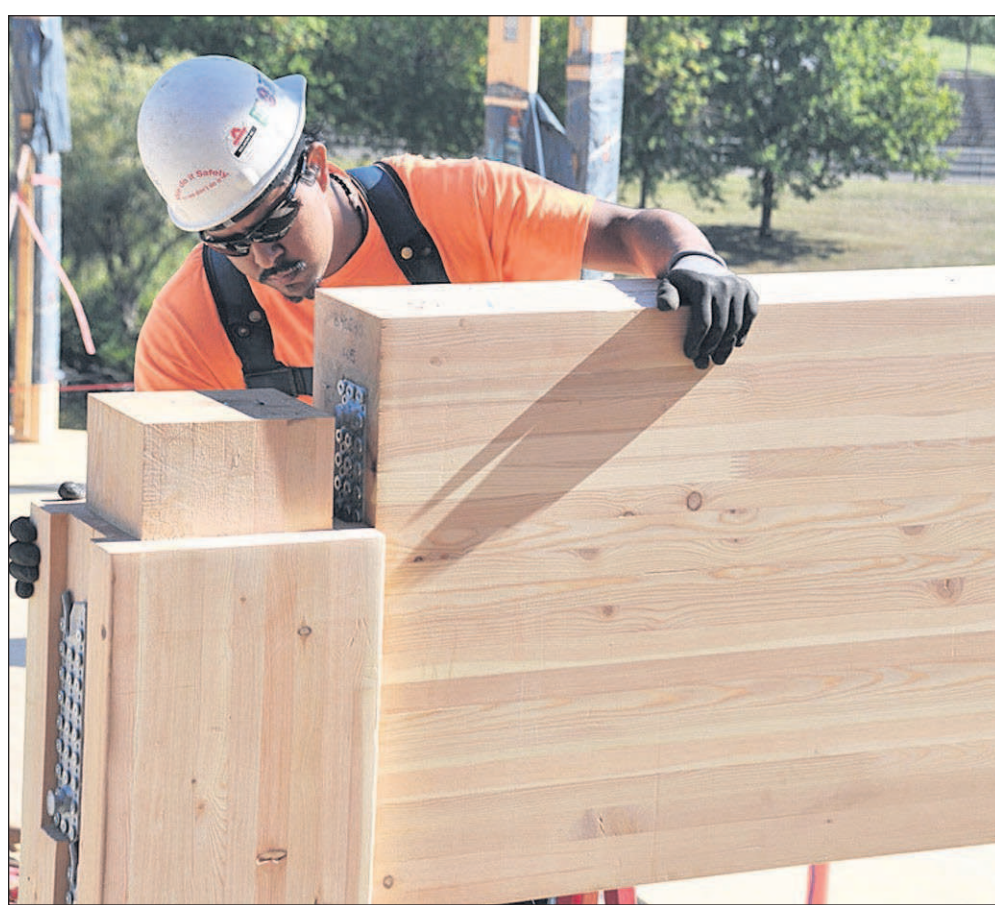
Capital Press File A worker guides a glulam beam into place Oct. 3, 2017, during construction of the First Tech Credit Union headquarters building in Hillsboro, Ore. The federal Timber Innovation Act would establish a research and development program under the USDA for mass timber products in building construction.
