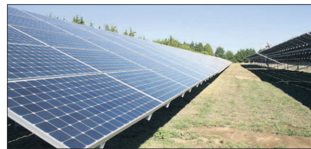
Capital Press File A solar project featuring honeybees in Oregon's Clackamas County is being appealed by farmland conservationists.
