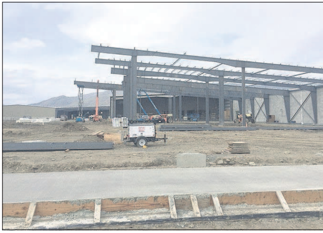
Courtesy of Allan Bros. Inc. Part of the new $40 million Allan Bros. Inc. apple packing and storage plant near Naches, Wash., in its initial construction phase last April.
