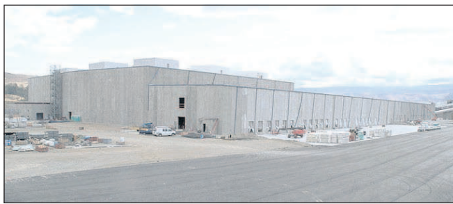
A new 479,000-square-foot, highly automated fruit storage and shipping center is under construction at Stemilt Growers, Wenatchee, Wash., on Oct. 13. The facility will be able to store almost 1 million boxes of fruit and ship them with few workers needed.
