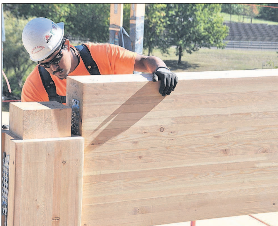
Eric Mortenson/Capital Press A worker guides a glulam beam into place Oct. 3 during construction of the First Tech Credit Union headquarters building in Hillsboro, Ore. The building, which will be five stories tall and include 156,000 square feet of office space, is believed to be largest U.S. structure so far built using advanced lumber products such as cross-laminated timbers (CLT) and glulam beams, posts and flooring. Advocates believe such wood products can replace concrete and steel in modest high-rises, and revive Oregon’s timber industry.
