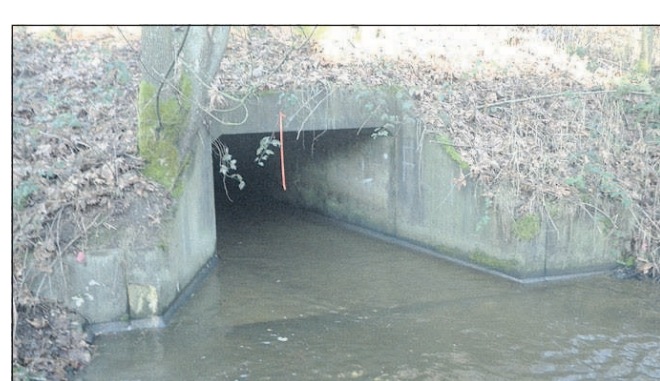
Church Creek flows through a culvert under State Route 532 in Snohomish County, Wash., in 2013. Washington Attorney General Bob Ferguson has appealed a federal court order to remove more than 800 fish-blocking culverts.
