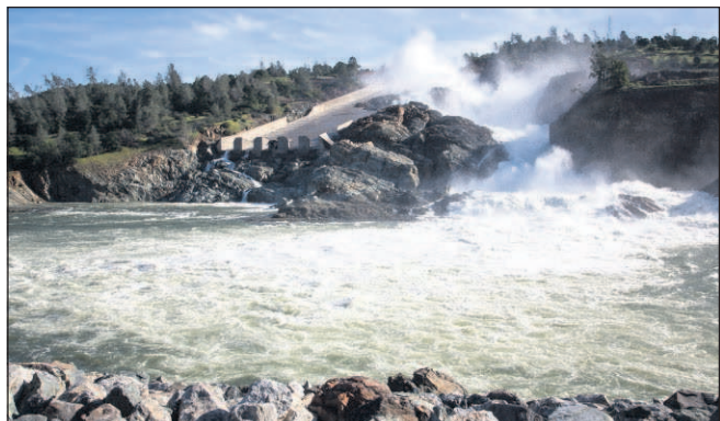
Dale Kolke/Calif. Department of Water Resources Water rushes into the diversion pool from a damaged Oroville Dam spillway. Repairs of the spillways continue.
