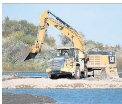
Courtesy of Idaho Power
