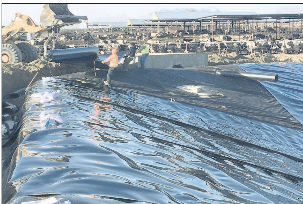
A worker rolls out the first of two 60 mil synthetic liners in a Cow Palace Dairy lagoon near Sunnyside, Wash., in early December.
