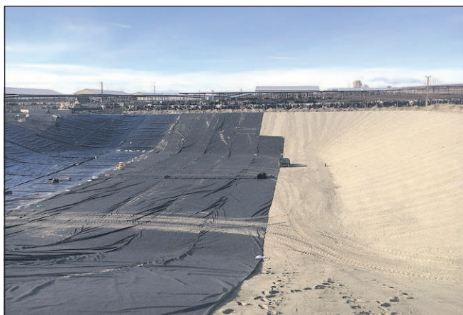
A Cow Palace Dairy storage lagoon is rebuilt in early December near Sunnyside, Wash. The cloth layer is in the center, and the first synthetic liner is at the far left. The system is intended to detect and prevent any leaks.
