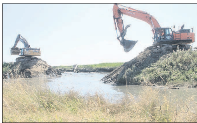
Excavators breach a dike earlier this year in Skagit County, Wash., to expose 131 acres of former farmland to Puget Sound salt water for fish habitat. A much larger effort is contemplated in a plan to flood thousands of acres of farmland bordering Puget Sound.
