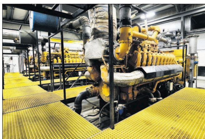
The three 2,000-horsepower engines in the powerhouse of the methane digester can produce 4.8 megawatts of electricity.
