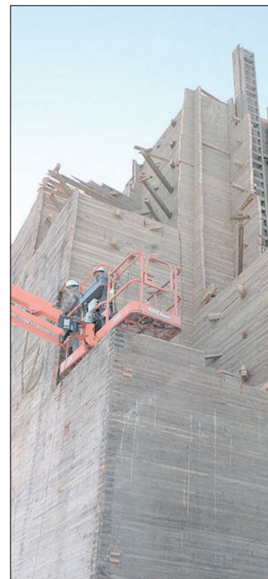
Workers from Northwest Reclaimed Wood, a deconstruction company, dismantle a grain elevator in Suver, Ore. Old wood from barns and other farm buildings is popular among woodworkers and home renovators.
