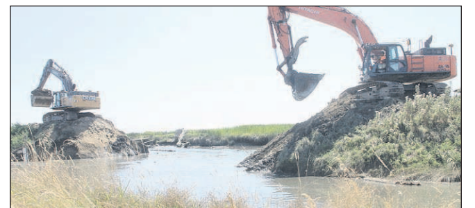
Excavators breach a dike Aug. 1 in Skagit County, Wash., to expose 131 acres of former farmland to Puget Sound salt water to create fish habitat.
